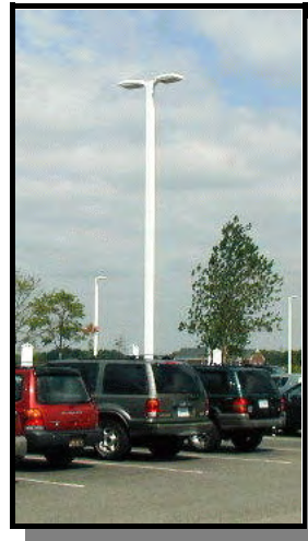
Parking lot light fixture
